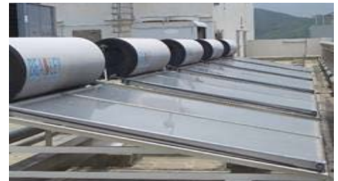
Solar hot water system installed at Lamma Power Station in Hong Kong.
