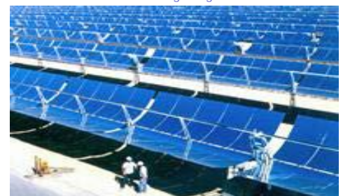
Concentrating solar power plant in the Mojave Desert, California, USA. Courtesy: DOE/NREL Credit: Gretz, Warren
