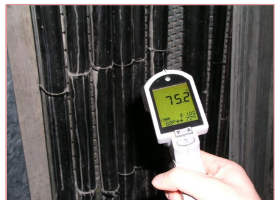
Overheating of Wiring
