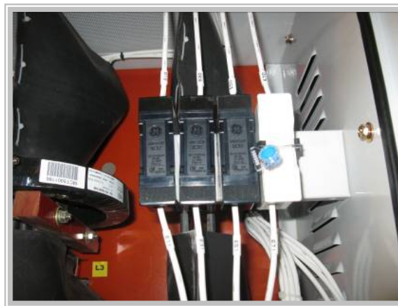
Figure 7 – Voltage Fuses and Link Inside C.T. Chamber
