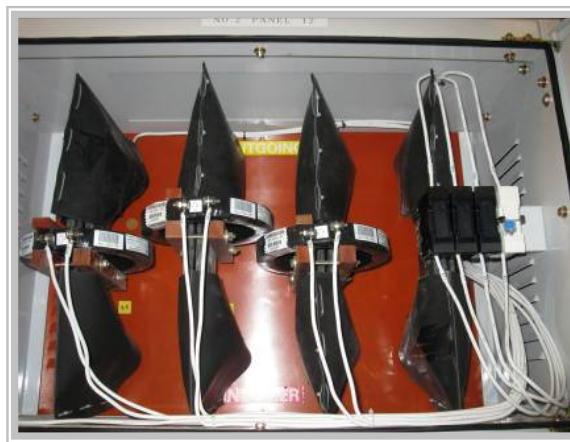
Figure 6 – Bare Busbars inside C.T. Chamber Insulated by Heat-shrinkable Materials
