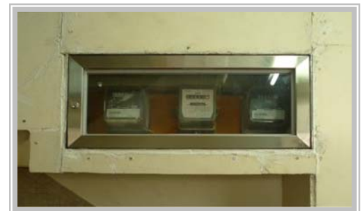
Figure 6 – Meter Cubicle / Enclosure
