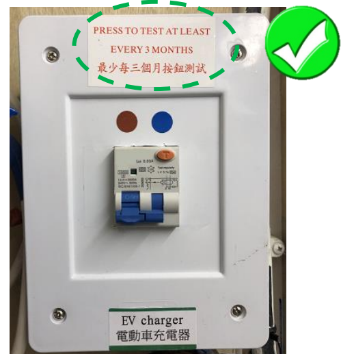
“Press to test at least quarterly” and “最少每三個月按鈕測試” notice should be provided at or near a residual current device.
