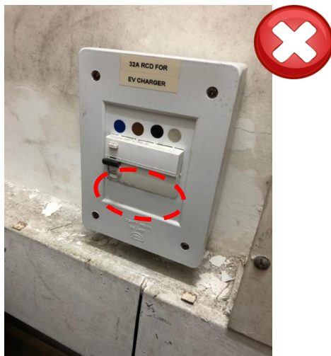
Notice of testing is not provided at or near a residual current device.
