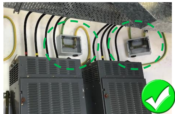
INSULATED ENCLOSURE COMPLETE WITH SCREW FIXED COVER AND A BILINGUAL LABEL: 接駁香港電燈有限公司接地系統與大廈總接地系統的接駁導線切斷連接 - 切勿移去 "Isolating Link for Bonding Conductor Between HK Electric Earth System and Building Main Earth System - DO NOT REMOVE"
