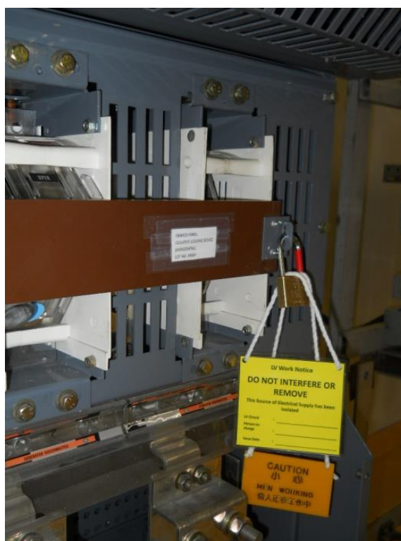
Figure 2: Locking and Caution Notices affixed to the disconnecter of LV isolator panel
