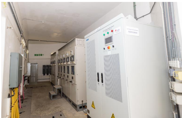
The LVDC power cabinet installed inside the distribution substation will further enhance the reliability of power supply to critical facilities at Ocean Park.
