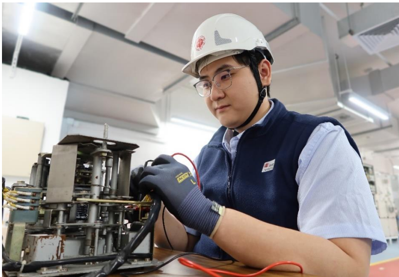
Mr. Zion Yung enjoys repairing electrical appliances at home, and now he is responsible for inspecting and maintaining switchgears in substations, turning his interest into his profession.
