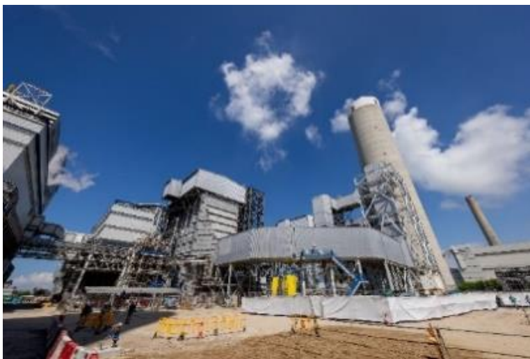
Unit L12 at LPS began commercial operation in end March 2024.
