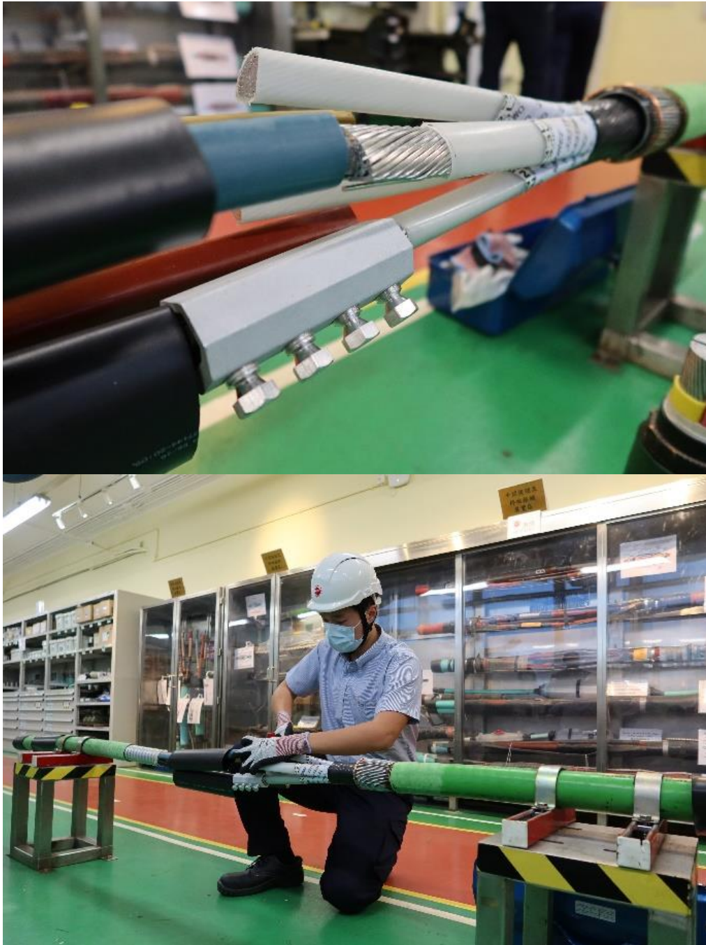
The AI-based Cable Health Condition Monitoring System conducts cable health diagnosis by analysing operational data of underground cables, helping engineers to formulate a repair solution.
