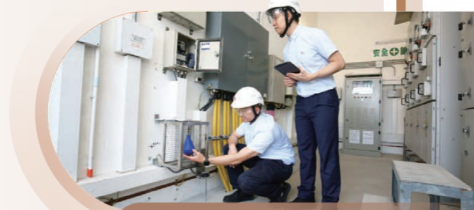
Enhanced flood-resilience measures at substations
